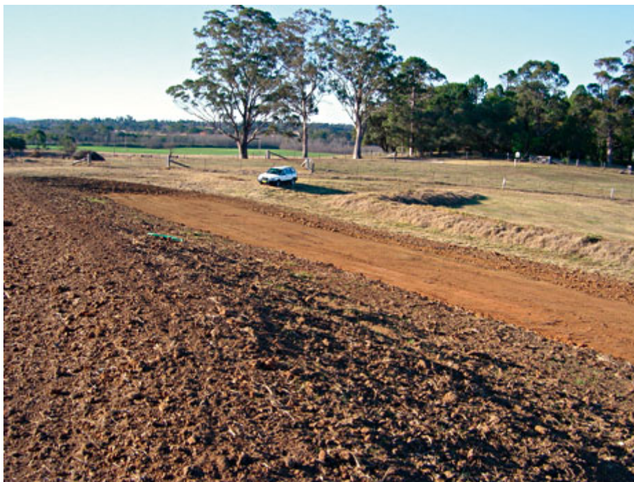
Figure 22. Area of CROA where vegetation and topsoil has been removed in preparation for the establishment of runoff plots (Blocks 2-4).
